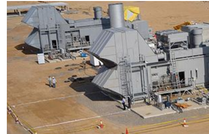
Al Hamra I 45 MW OCGT First aeroderivative GTs in Ras Al Khaimah, UAE, built on fast- track
