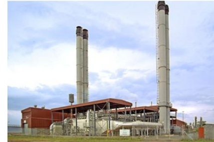
Newcastle Cogeneration 18 MW CHP Syn Gas First IPP in South Africa, KwaZulu Natal
