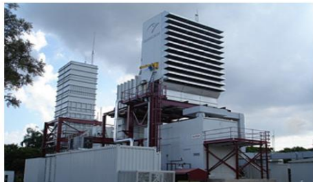
Guaracachi O&M > 500 MW of gas-fired capacity in Bolivia Installation of new OCGT and CCGT capacity > 300 MW
